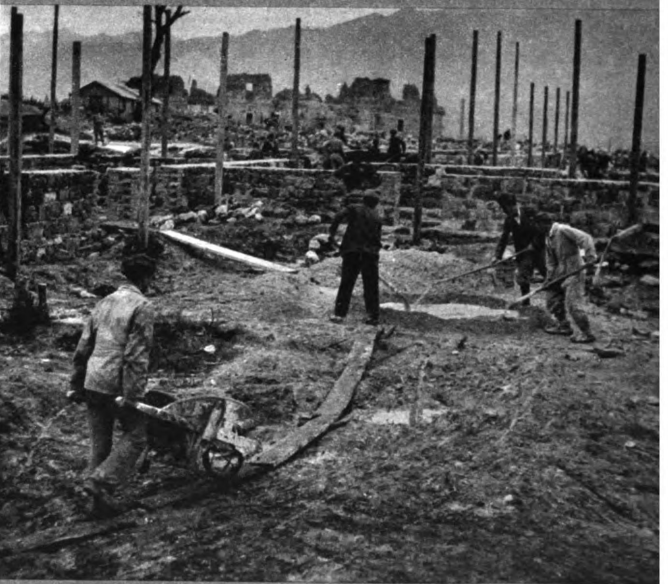
A new Cassino has started, 1 1/2 miles northwest of the old one. Italian laborers are working on a group of 150 one-story houses.
