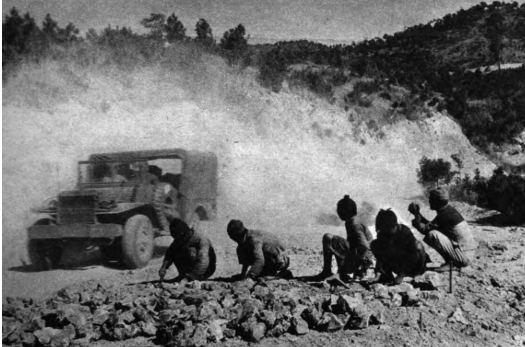
9 Chinese laborers work slowly and patiently to build a stone surface on the road, fitting each rock by hand.
